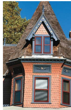
Images are framed to show surrounding elements and materials, and to demonstrate how various junctions are resolved, as with this complex octagonal turret and dormer.
